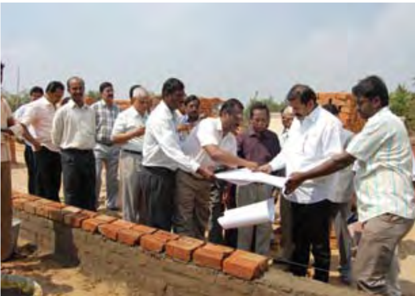
Hon'ble Minister Shri.D.Napoleon briefed by CPWD officials at the construction site of New Building, NIEPMD
