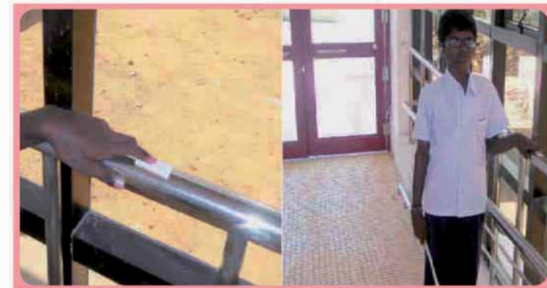
Tactile signage through braille
